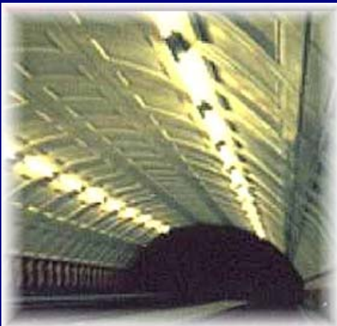
Fire retardant tunnel lining
